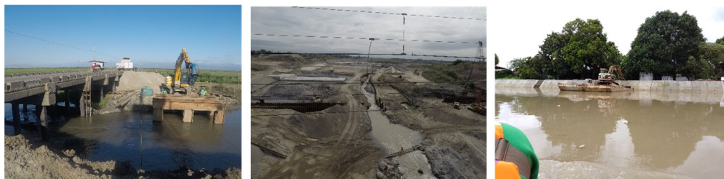
Figure 1. Example of river channel-improvement activities in the Pampanga River basin of the Philippines. (Photos: Mr. Hilton Hernando, Pampanga River Basin Flood Forecasting and Warning Centre).
