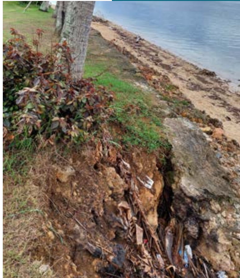
Collapsing seawall in Yadua village
