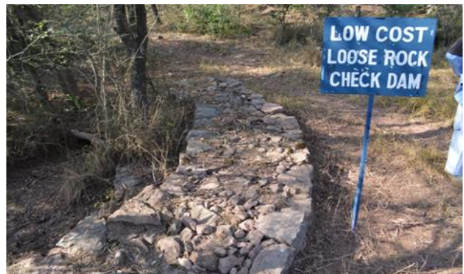
Figure 1: Loose Rocks (Check Dam)
