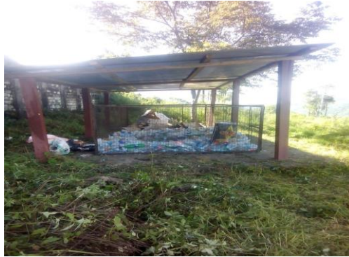
Figure 6.3 Recyclable storage facility
