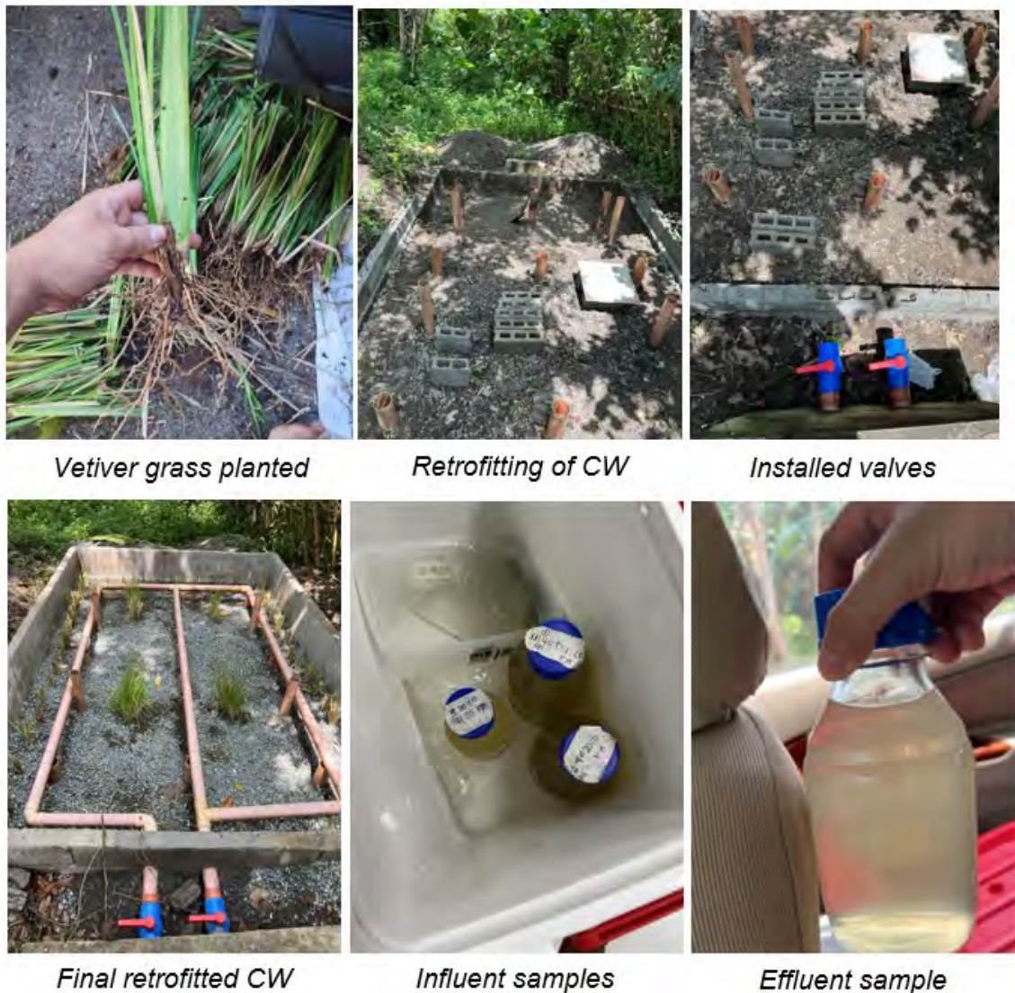
FIGURE 8. Retrofitting and sampling activities carried out at the CWs in the Green Village.
